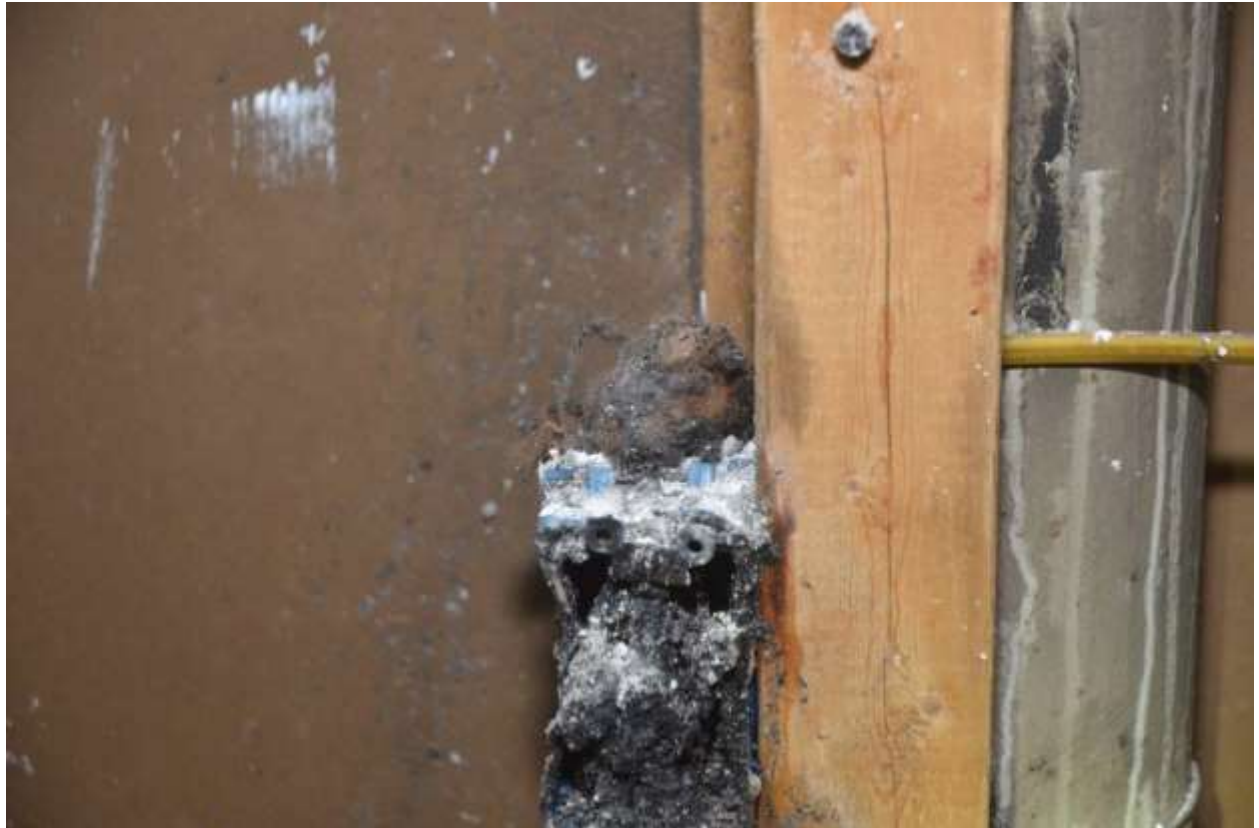
468 Thomas Ave.Fire Dwelling Photos 11-18-23
